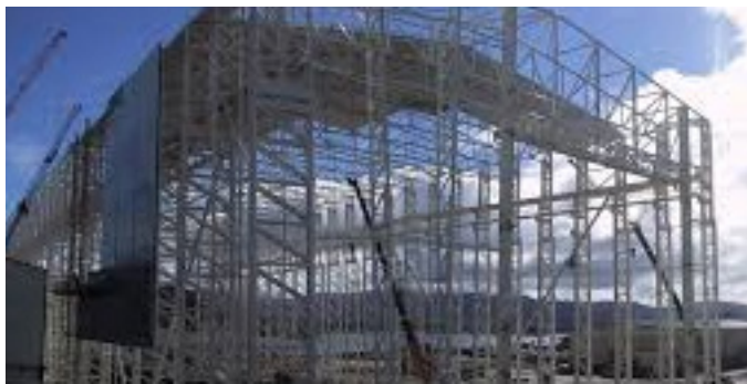
Fabricated structural steelwork must be CE -marked from 1 July 2014.
