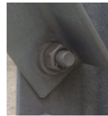
On the nut side, where a washer is used, there are no cracks.
