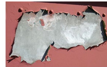
Figure 1 Peeling paint from galvanized door
